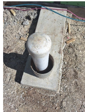
Well with steel sleeve, but annular cement does not reach the top of the steel sleeve- this can cause the cement to crack or
