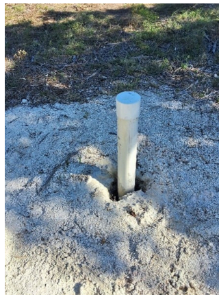
Well with no steel sleeve- essentially an open hole into the aquifer that can allow contaminants to enter.
